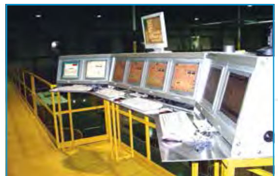
The entire line can be remote-controlled via a central operating terminal, minimizing staff input. Current production status can also be monitored at any time.
